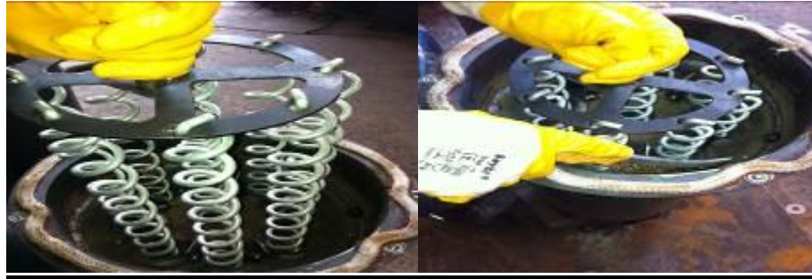
Cleaning of the suction fan and the flue tube
